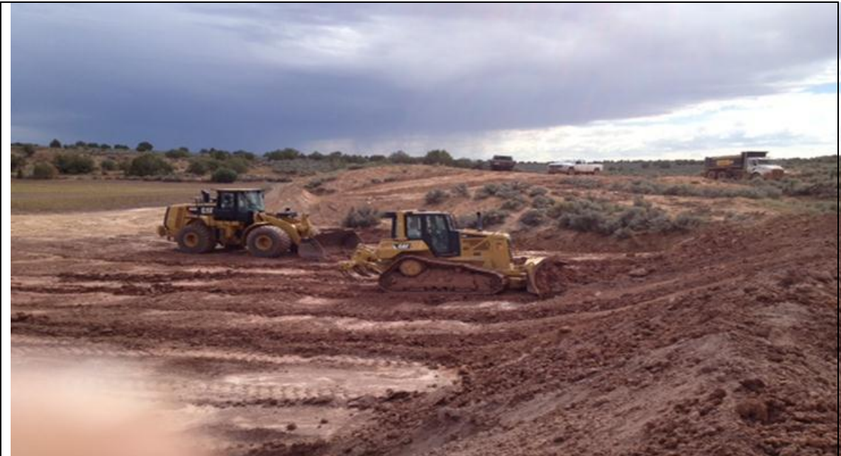
Equipment moving sediments from behind dam (off left of photo) to construct a “spreader dam” to keep work area dry during runoff/winter.
