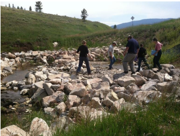
Rock below fish passage culvert along Highway 191
