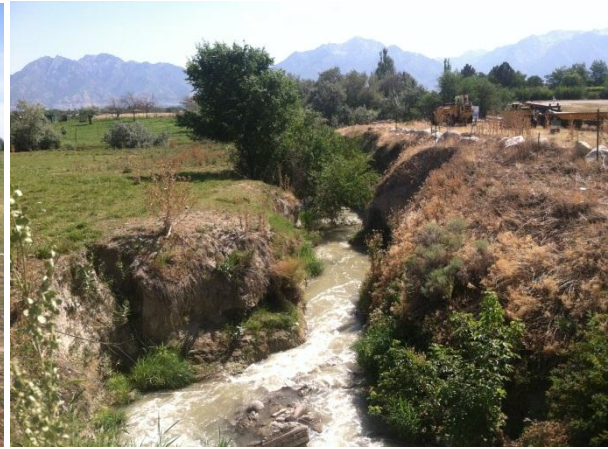
Erosion from Culvert on Bingham Creek
